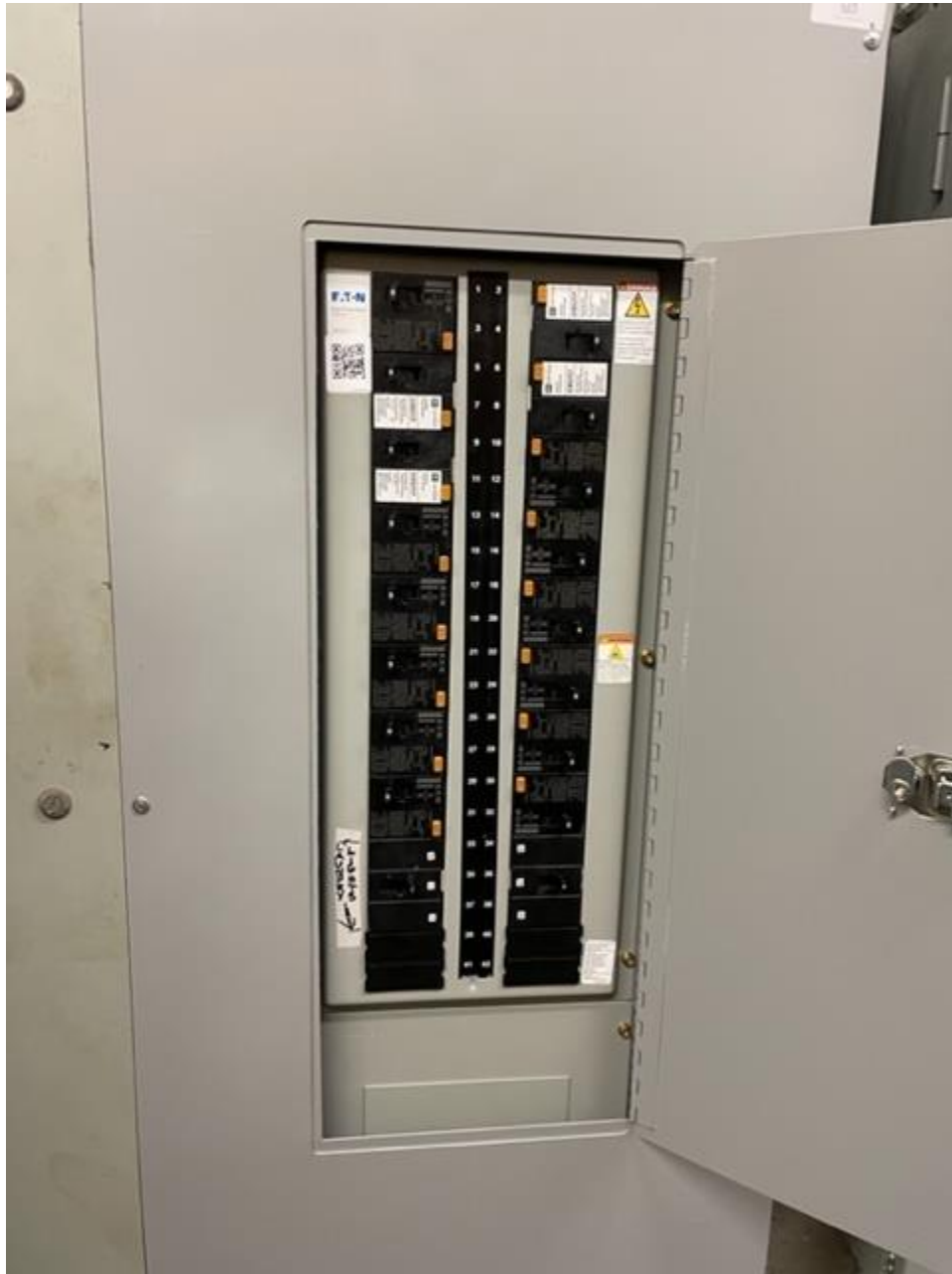
New GL Panel Installed Circuits to be switched back over 15 March 2022
