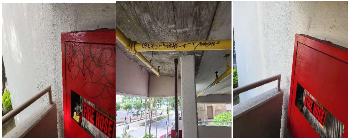
Graffiti 2 nd Floor Tower 1 Parking Garage
